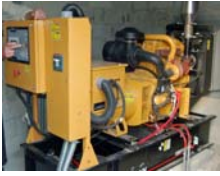
Generators can cause major problems when not properly wired.
